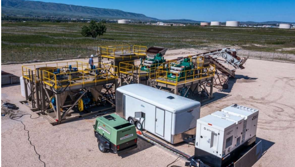
Figure 5: Gen B continuous on-site remediation HPSA system.
