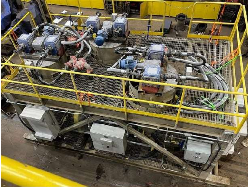
Figure 14: Gen B installed at a phosphate mill.
